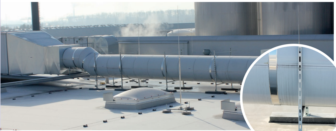
Ventilation system (air volume total 430,000 m 3 )
