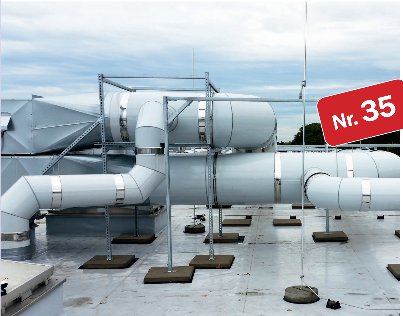
Ventilation system (total air volume 9,400 m 3 )
